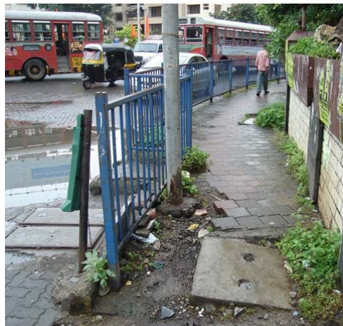
Fig. 1: Compromised pedestrian convenience
